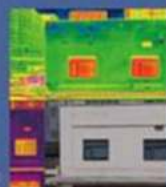
Seepage in R1 and R4 Bulging in R2 and R3
